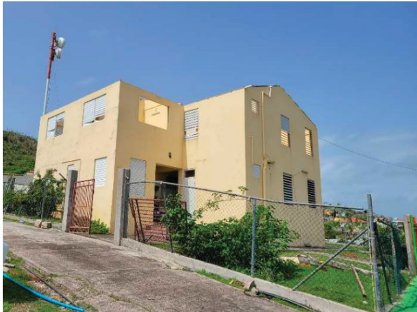
Complete loss of its roof structure in the Petit Martinique Medical Station , the only one serving the island (600-800 persons). Healthcare services were restored with the support of trucked water and small generators. Photo PAHO 2024
