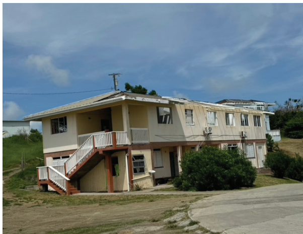
Nurses' housing at the Princess Royal Hospital severely affected in its roofing structure. Photo PDNA team.
