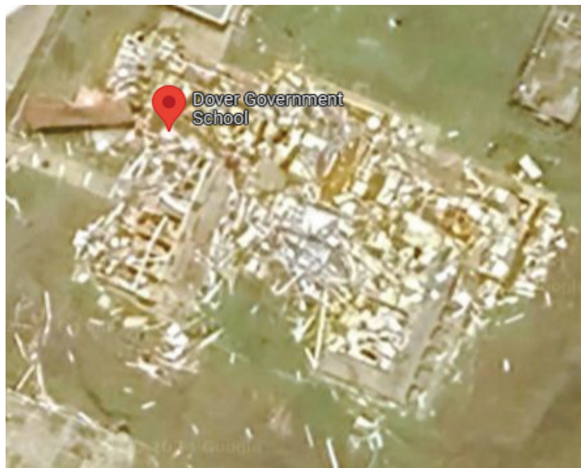
Figure 16: Dover Government School After Hurricane Beryl
